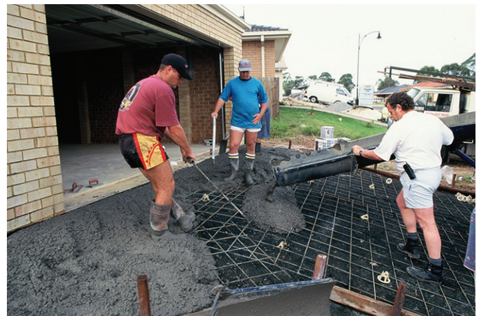
Example of inadequate bar chair placement in a residential concrete pavement.
