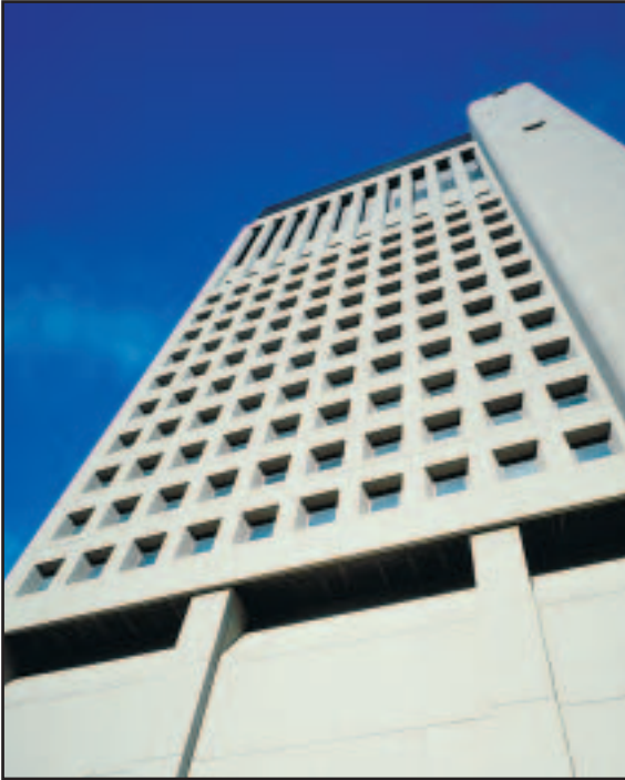
Commonwealth Bank Building, Sydney – an example of a high quality, durable veneered facade
