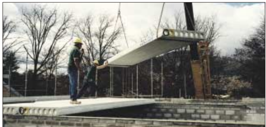
Erecting 200 mm 8 m span hollowcore planks on loadbearing blockwork at a townhouse development in Braddon, ACT
