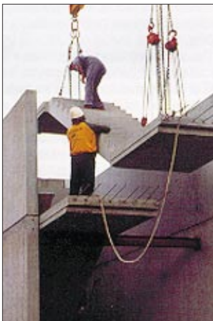
Locating precast stair flight and landing; use also of precast core walls
