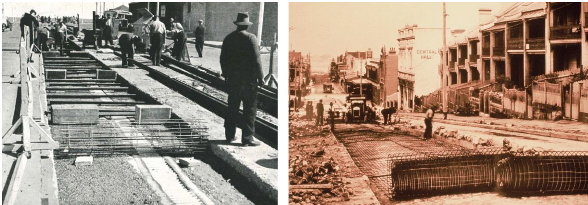
Figure 3 Rolled mesh used on Melbourne tram track foundation (left) and Walker Street, North Sydney (right)
