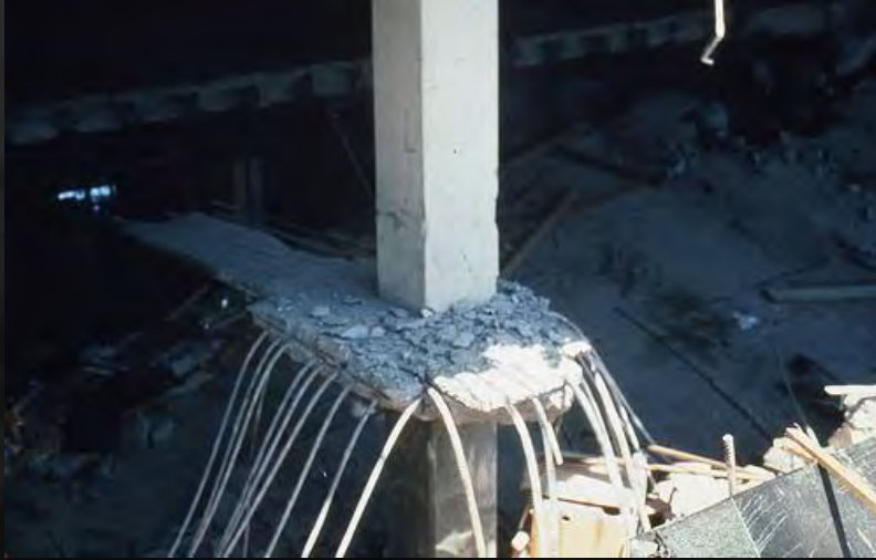
Remains of car park floor – Old Newcastle Workers Club NSW - Brittle failure & progressive collapse (Photo courtesy Cultural Collections, The University of Newcastle, Australia)
