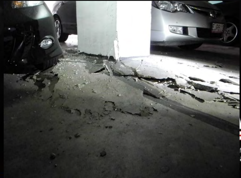
Punching shear failure Hotel Grand Chancellor Christchurch, NZ
