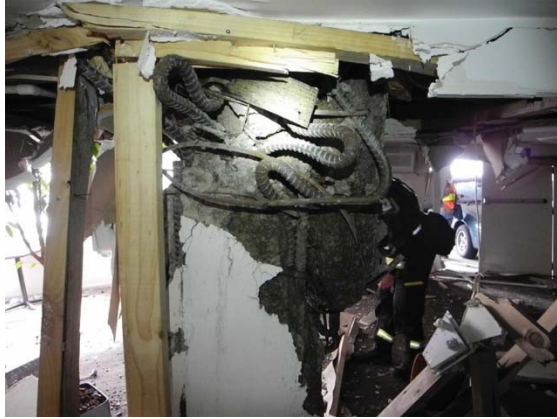
Figure 4: Failure of column at the Hotel Grand Chancellor, Christchurch due to poor confinement, (Photograph courtesy Peter McBean)
