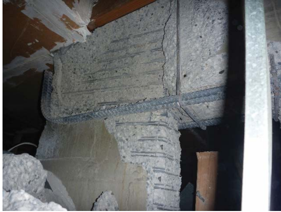
Figure 3: Failure of Beam/Column connection. Copthorne Hotel, Christchurch (Photograph courtesy Peter McBean, Wallbridge and Gilbert)
